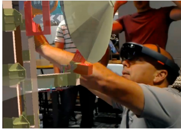
Figure 1. HGA XR installation rehearsal. The team used XR to rehearse the installation steps described in a work instruction document and discovered several “gotchas” during the process, leading to revisions that improved the instructions.
